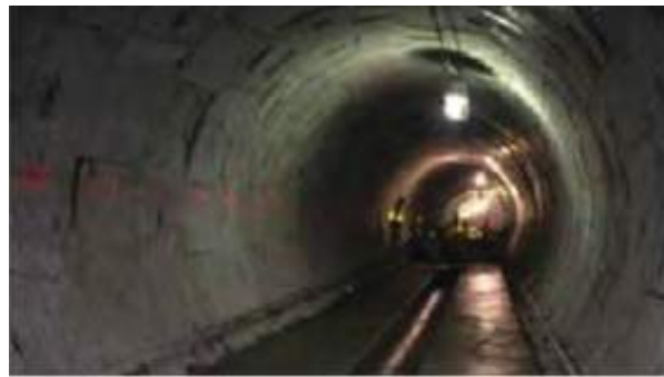
Storage Tunnels (Grey Infrastructure)
